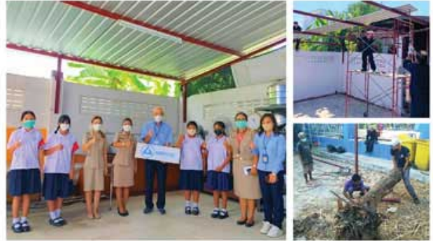
METCO2 Build a clean canteen promote safety care for the environment. (At Wat Saothongnok school)
