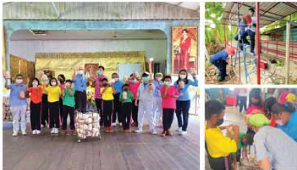
METCO3 Learning support and renovate a mushroom growing house. (At Wat Bua Roi)
